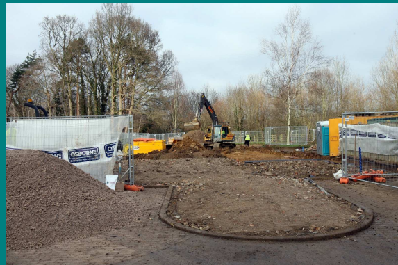
Saxon Weald is creating 22 new affordable homes after combining two small redundant plots.
